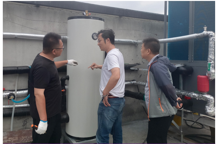
Integrated "57kW Photovoltaic and Thermal" heating system for office/industrial building
