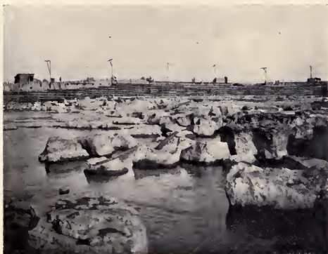
A Portion of the Unwatered Area The Electrical Development Company of Ontario, Limited
