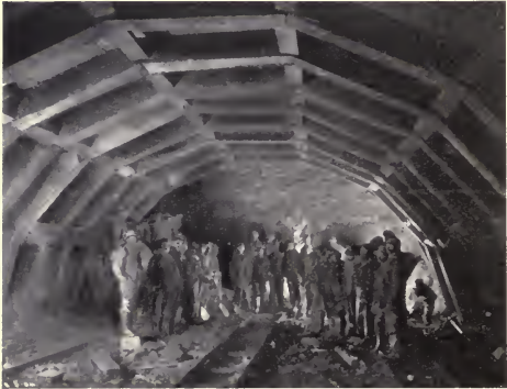
Main Tail Race Tunnel Above Spring Line The Electrical Development Company of Ontario, Limited
