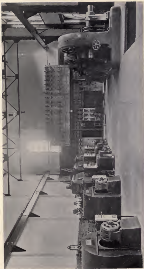
Virginia Street Substation, Buffalo—The International Railway Company
