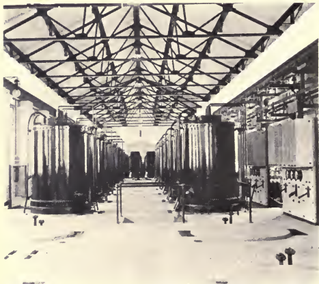
The Step-Up Transformer Plant of The Niagara Falls Power Company, Containing Transformers Having Aggregate Output of 60,000 H. P.
