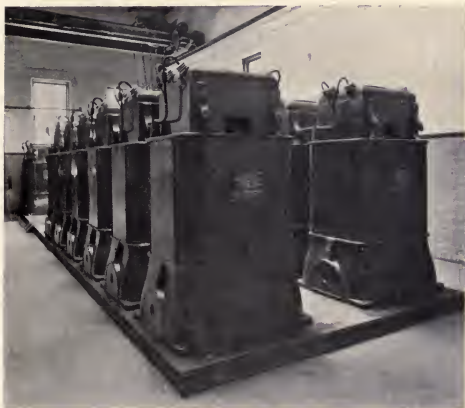
Transformer Room, Wilkeson Street Substation The Cataract Power and Conduit Company
