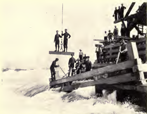
Constructing Cofferd Dam at the Cascade The Electrical Development Company of Ontario, Limited
