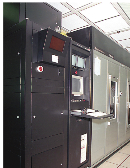
The world's first full-field step-and-scan 193-nm lithography system, built by SVG Lithography, was installed in Lincoln Laboratory's cleanroom facilities in 1993.
