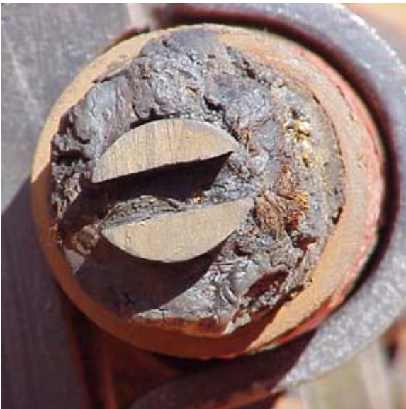
figure 6. Original Edison two-wire dc distribution line showing the half-moon cross section of the conductors and the conduit and insulation used (photo courtesy of Robert Lobenstein).
