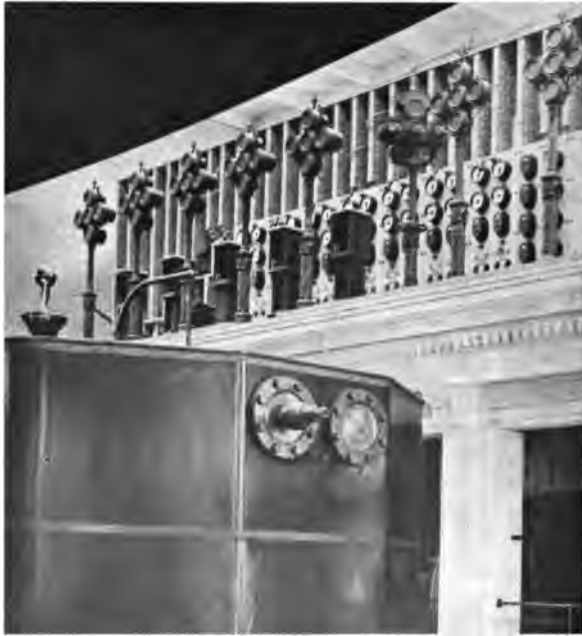
Fig. 7—Switchboard—Ashley Street Plant
