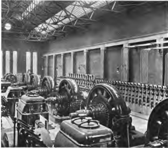
Interior Central Substation
