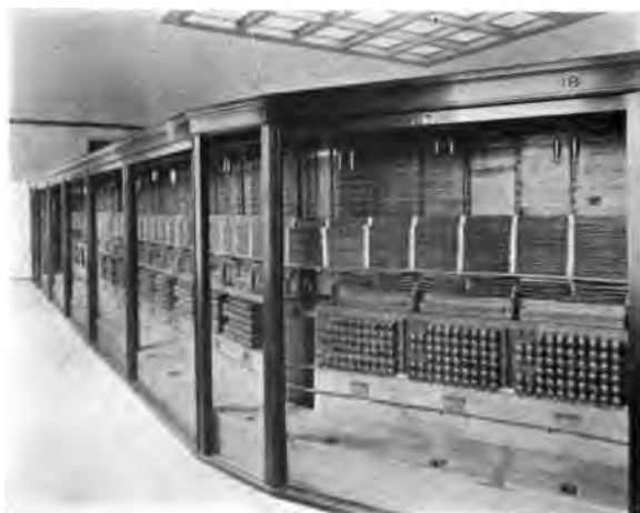
Rear View of Switchboard—Delmar Station
