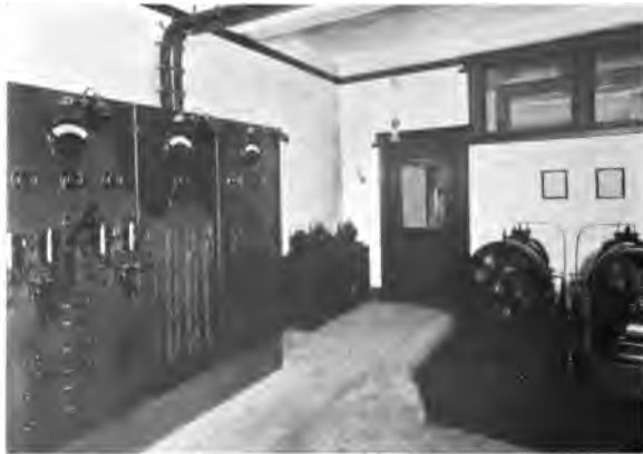
Power Room—Delmar Exchange
