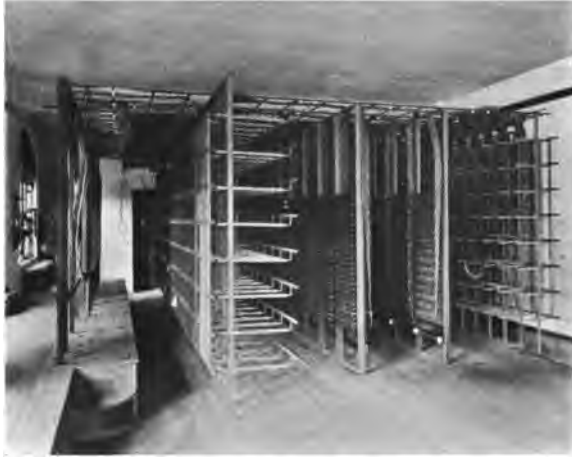
Distributing Room—Delmar Exchange
