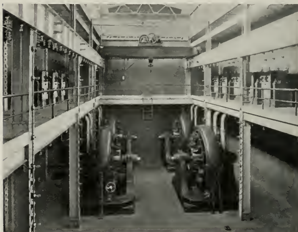
Interior of Substation Manhattan Division
