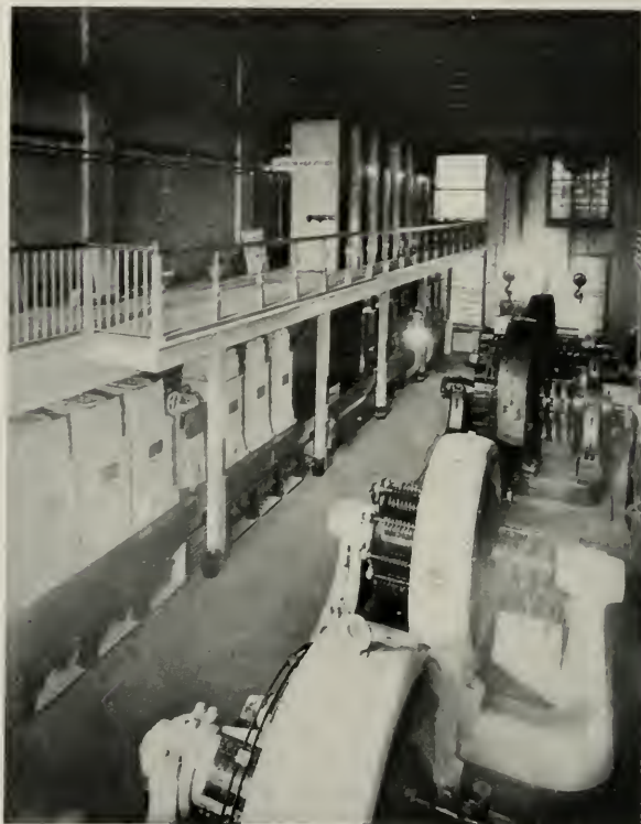
High tension gallery, 83rd Street Station
