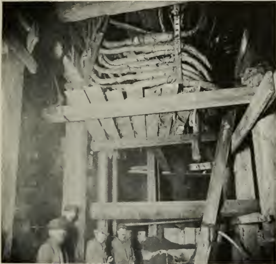
Cables at Broadway and Fulton Street before fire, manhole having been removed to make way for underground railway structure
