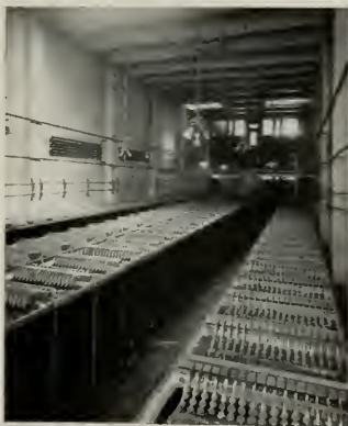
Battery room, Elm Street Station
