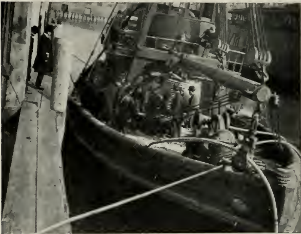
Cable tug laying a 30 pr. lead covered submarine cable under North River
