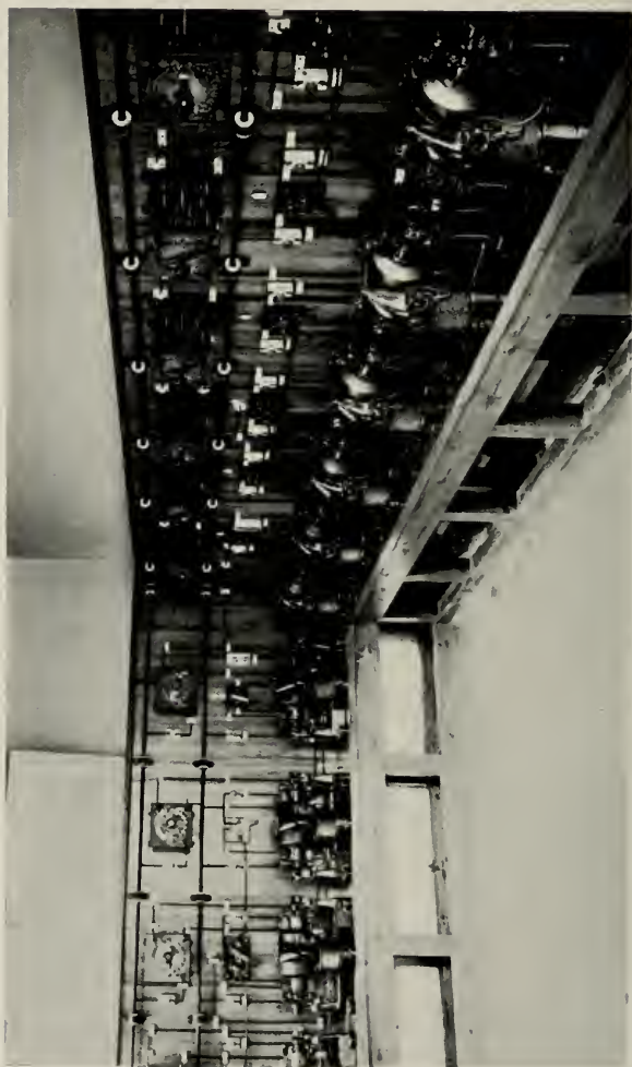
Motor Dynamo Plant
