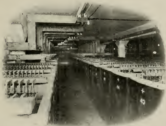
REPRESENTATIVE BATTERY ROOM
