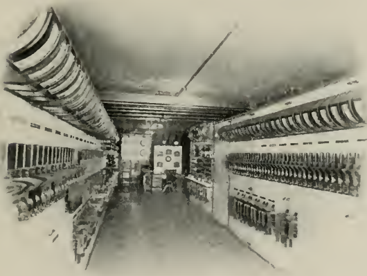
DISTRIBUTION ROOM, ADAMS STREET
