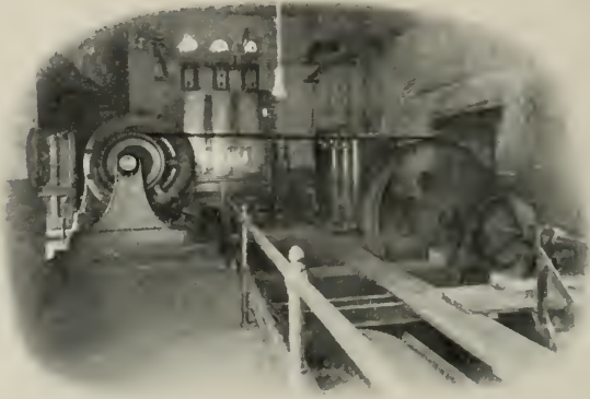
MOTOR AND CONNECTION, MAIN SHAFT OF BRIDGEPORT PUMPING PLANT
