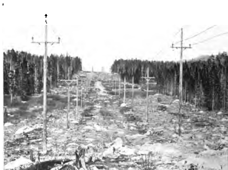
FIGS. 27 AND 28. MISSOURI RIVER POWER COMPANY'S TRANSMISSION LINES.
