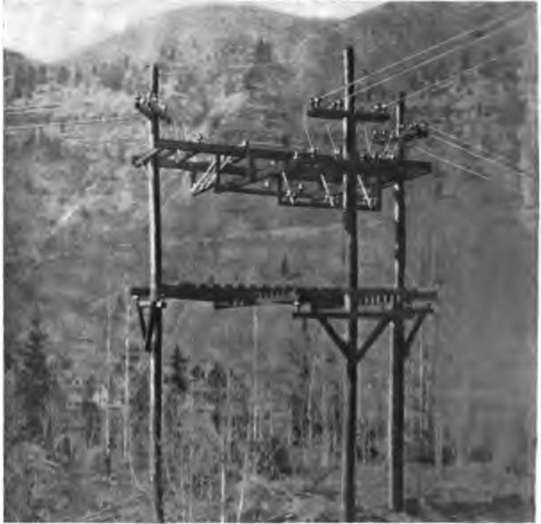
FIG. 2.— AN OPEN-AIR SWITCHING JUNCTION.
