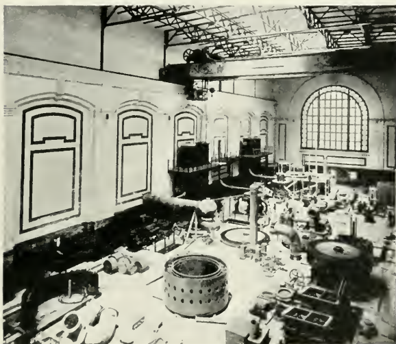
Turbine Station, Edison Illuminating Company
