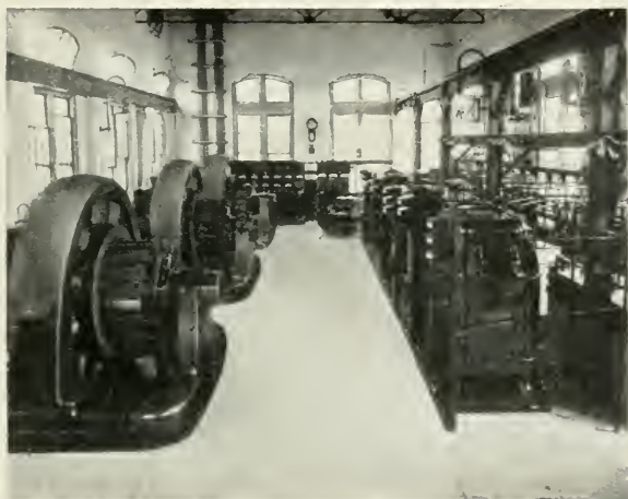
Interior, Brockton Sub-station
