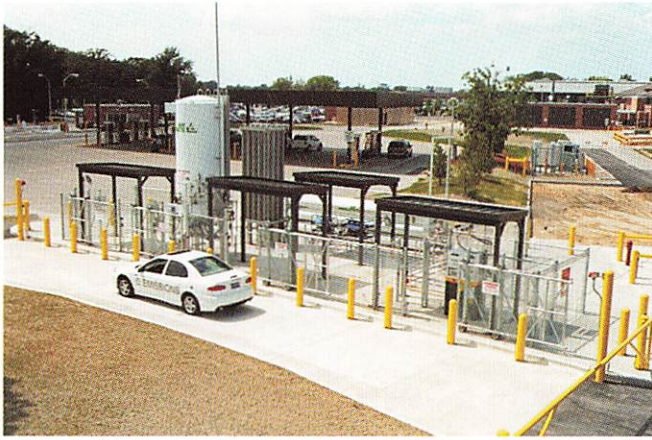
Figure 9 Ford Motor Company's liquid and gaseous hydrogen refueling station.
