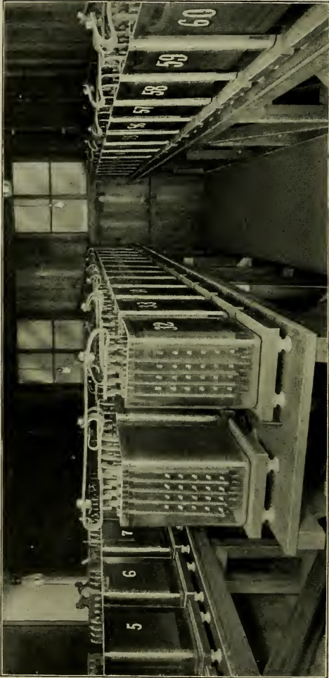
A Typical Installation of Chloride Accumulators for a Residence Plant
