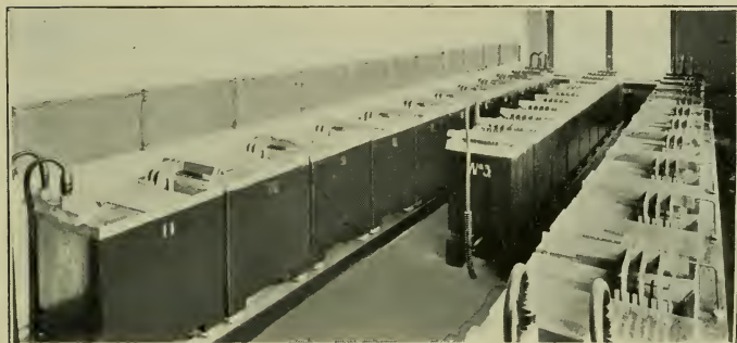
Battery Room, Main Exchange
