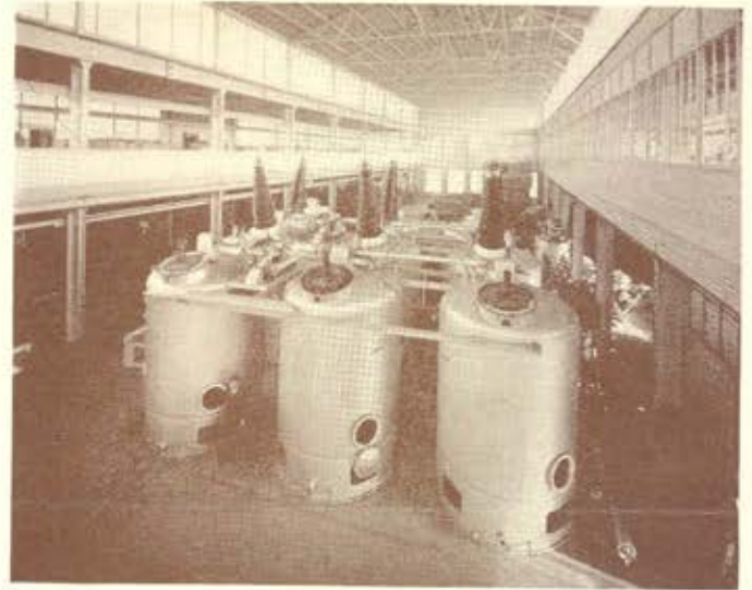
Oil Circuit Breaker Assembly Floor of Pacific Electric Manufacturing Company
