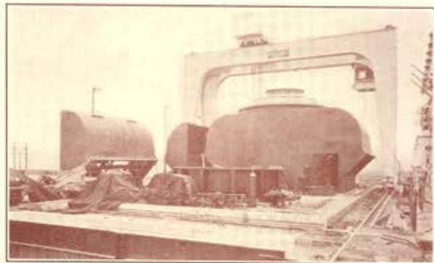
Leaside Station—25,000 kv-a. Outdoor Condensers
