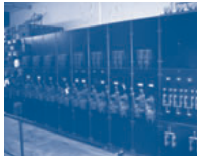
Dolgeville Mills Switchboard, circa 1910, copyright Dolgeville Mills
