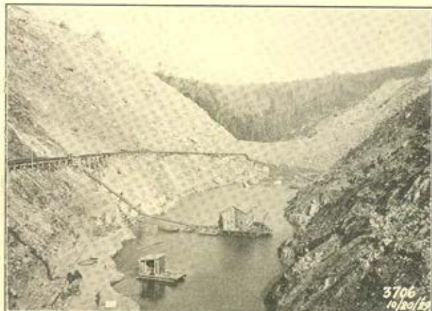
Sluicing Earth Dam for the Springfield Water Works and Cobble Mountain Hydroelectric Development
